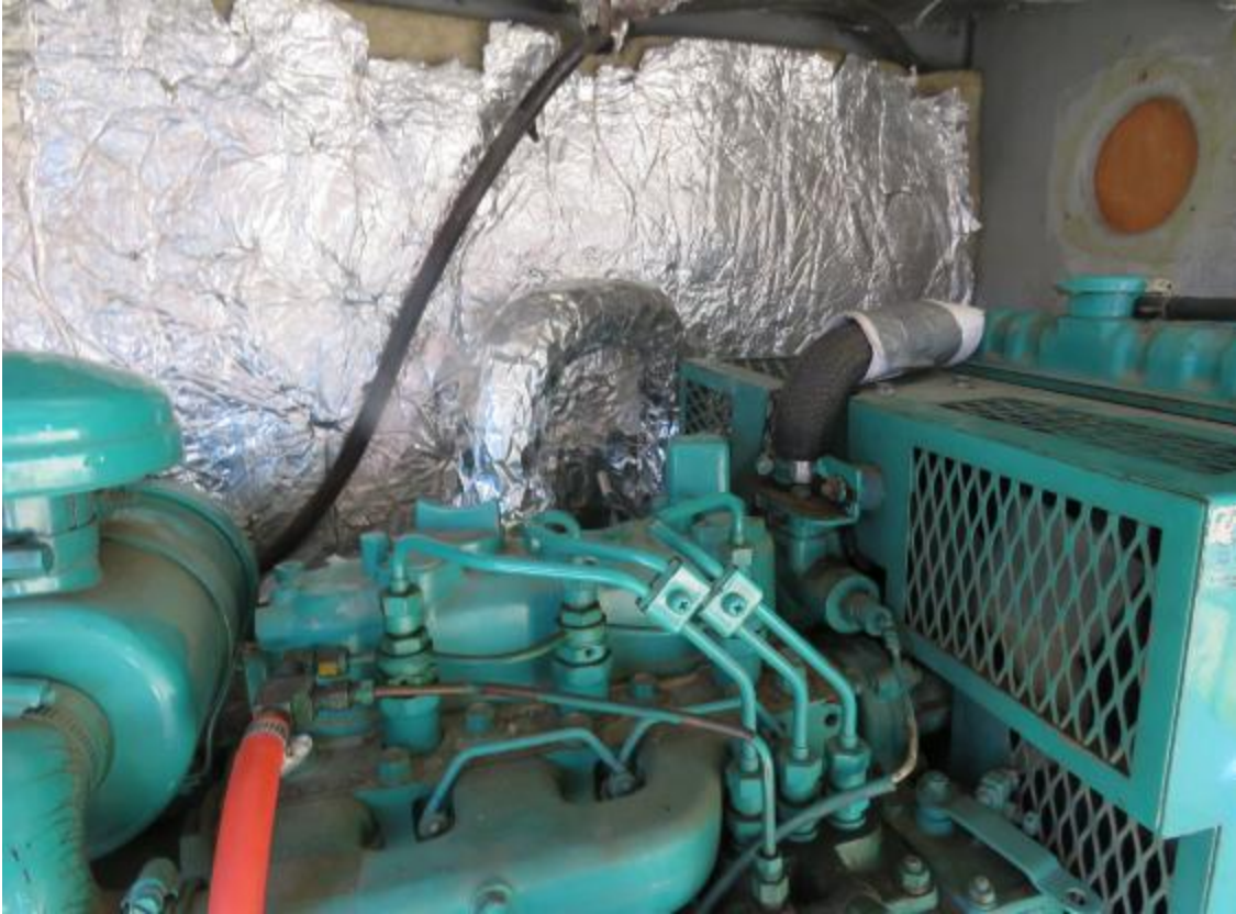
Top exhaust pipe after it is wrapped with foil as an added layer of protection.
