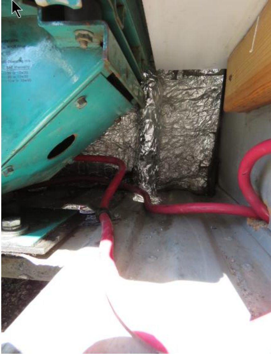
Wrapped exhaust pipe going through the floor.
